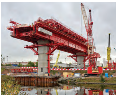
MSS 'Webster' on the first span of the south approach viaduct – October 2016.
