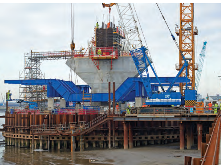
North pylon hammerhead – upper pylon first lift under construction; assembly of form traveller at cofferdam level.
